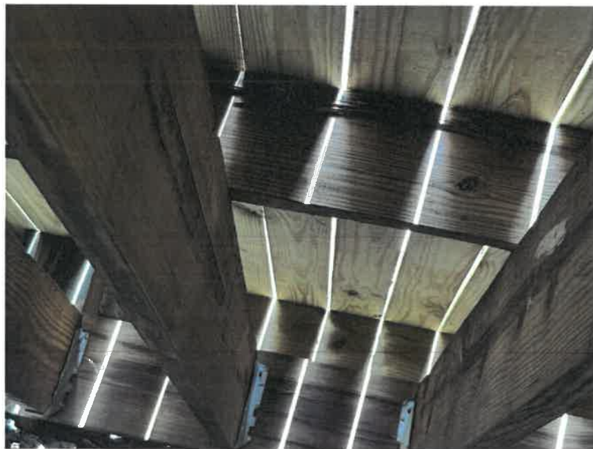
Photo 10. Screw improperly installed, minor deterioration of stringer
