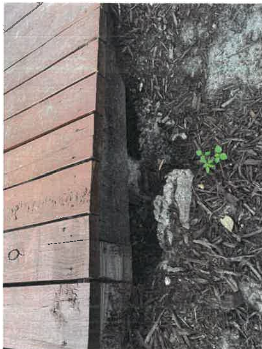
Photo 6. Undermining of boardwalk
