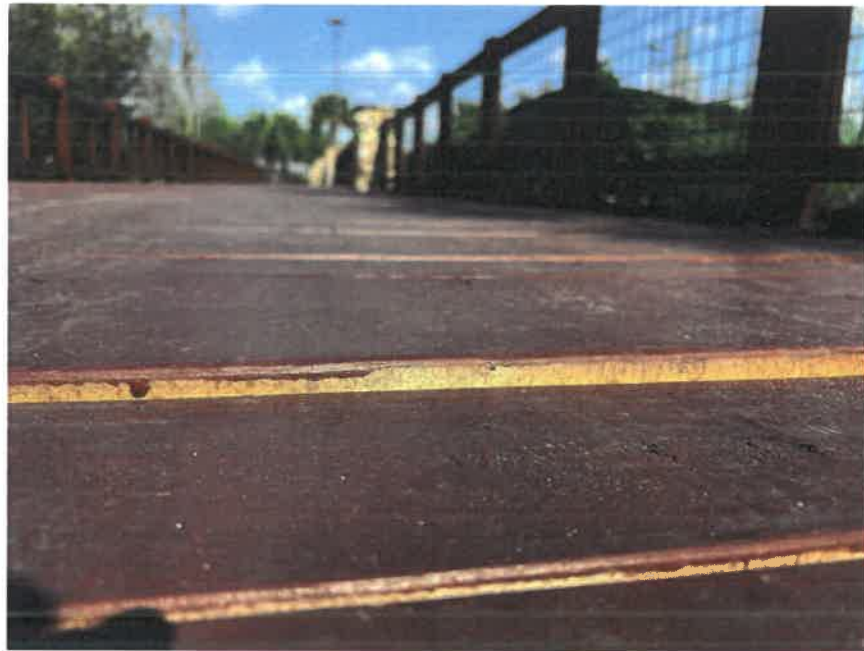
Photo 3. Vertical gap between adjacent boards
