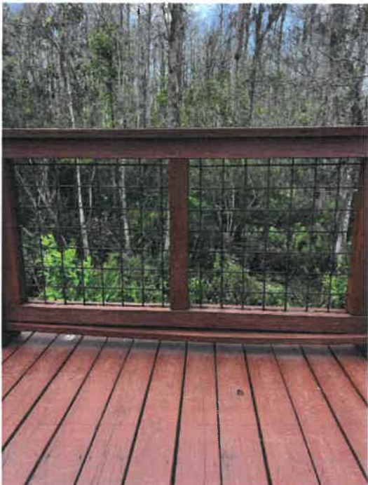
Photo 7. Sagging bottom rail
