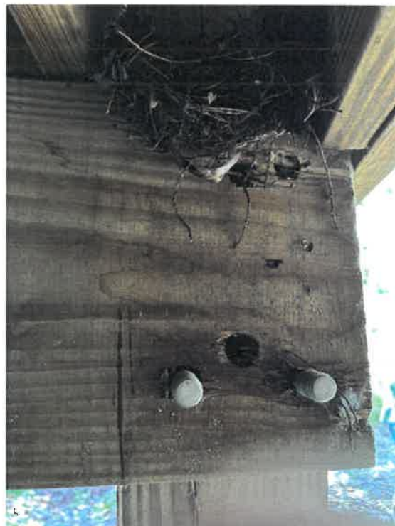
Photo 4. Missing bolts and nuts in fascia stringer to pile connection
