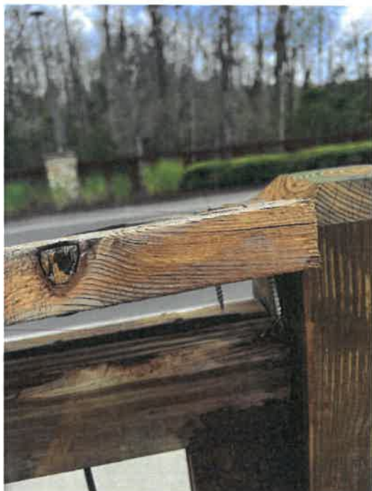
Photo 8. Top rail separation
